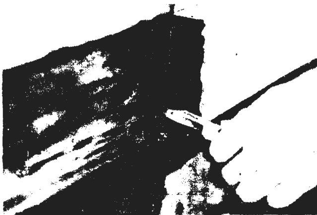
An example of decay—serious decay—in a stern timber.
